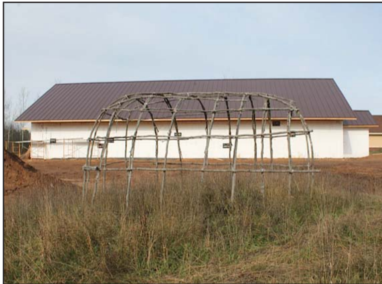
The new Big Drum building is on course for an official opening the second week of December.
